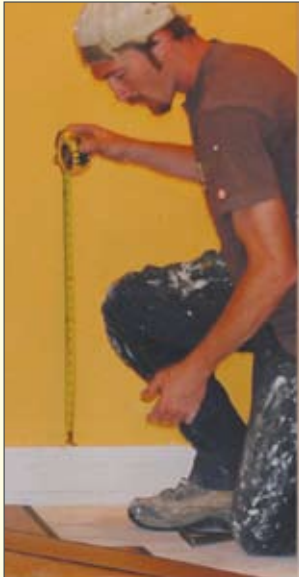
Kyle Smith lays flooring, one of the last steps in the completion of Janus House
